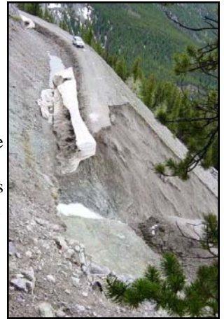
Road and mountainside washed away by the Grand Ditch breach. The ditch runs to the left of the road shown in the photo. Photo courtesy of James Sanborn, Rocky Mountain National Park.
